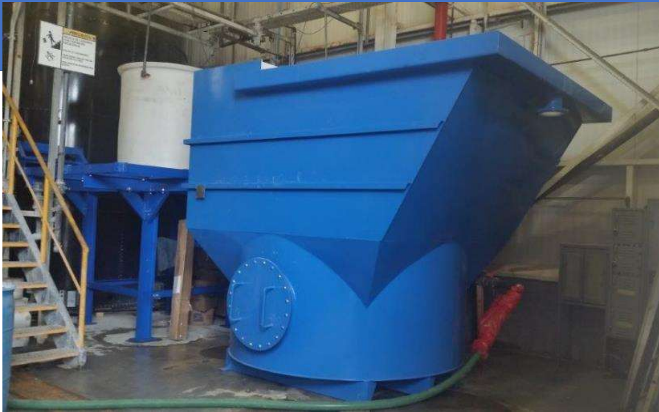
Component for water-treating plant
