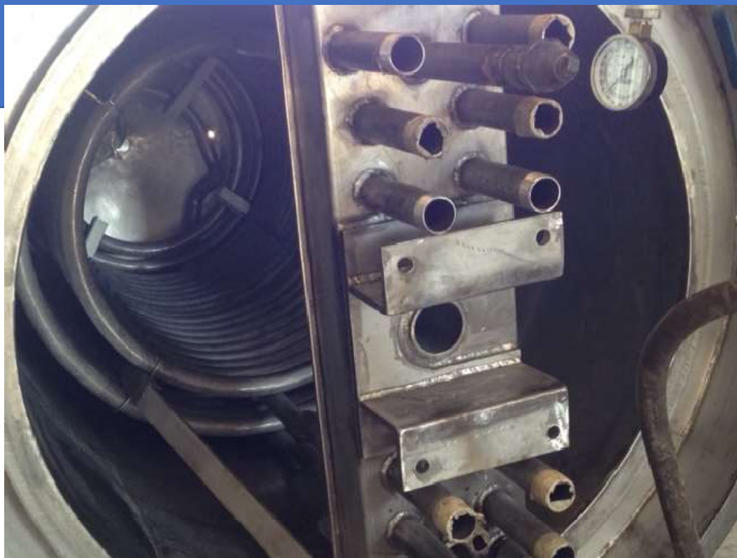
SS 2 Stir Reactor Tank with serpentine coil Chemical Industry
